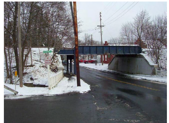
Low Vertical Clearance at RR bridge
