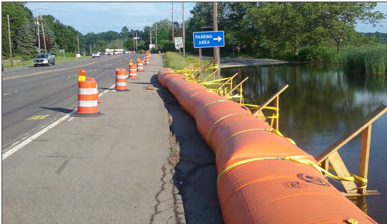
In 2017, a temporary dam was erected along NYS Route 404 (Empire Boulevard) at the southern end of Irondequoit Bay to protect the road from high water levels
